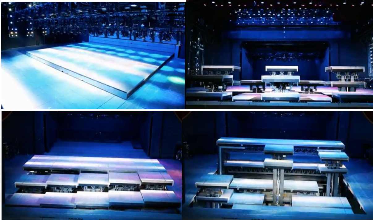
Fig 17, the stage elevator systems
