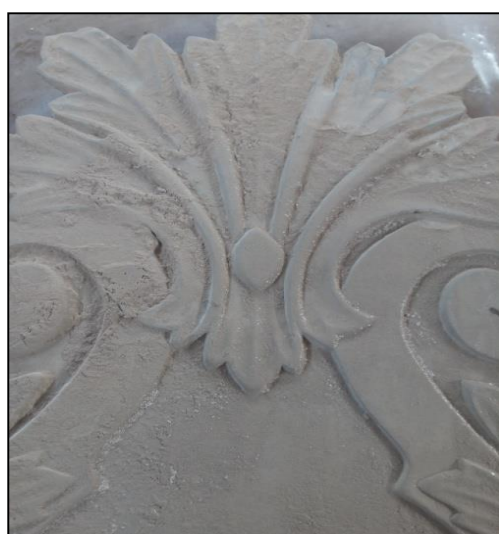
Figure 6. The heavy dust and dirt on the decorative unit
