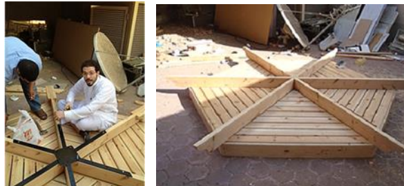
The figure shows the installation and assembly of the ceiling unit for the hexagon canopy. A metal assembly unit was created to be installed on both sides "above and below the ceiling beams.
